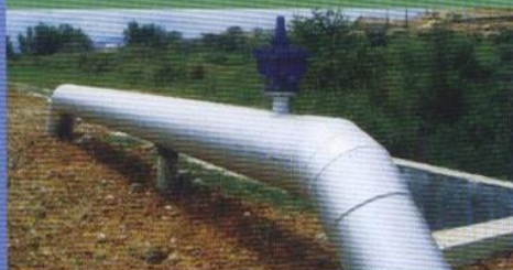
PIPE LINE S-BEND
