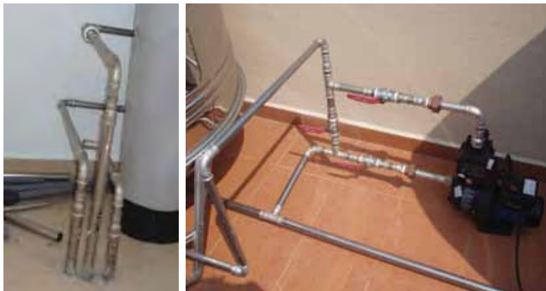
Pipes Connection at Water filter tank
