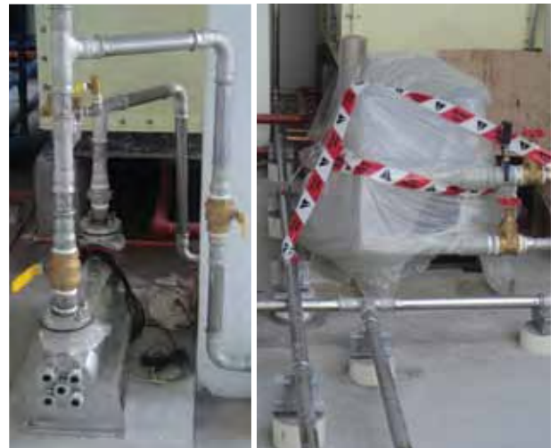
Pipes connection from Booster Pump
