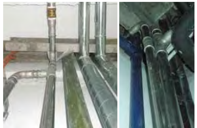
Riser Pipes for High Building
