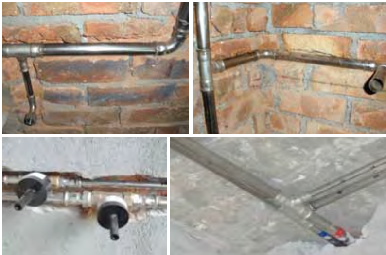
Internal Plumbing (Hot and Cold Water)
